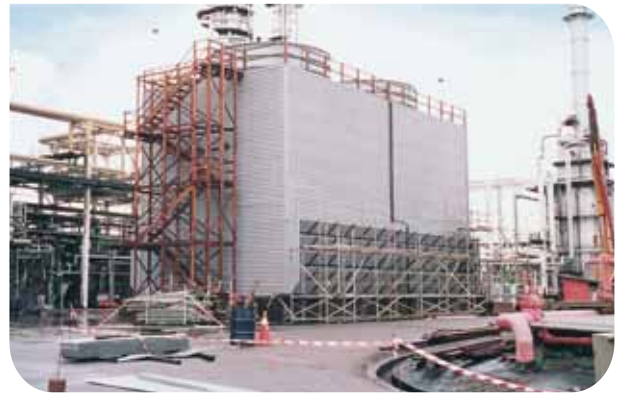
:: Esso Refinery Port Dickson Reconstruction, 3500 m 3 /hr (2 cells).
