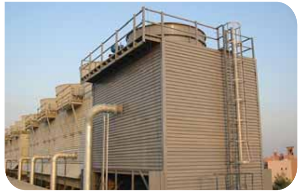
:: Ibn Battuta Gate Complex Dubai, 950m 3 /hr/cell.
