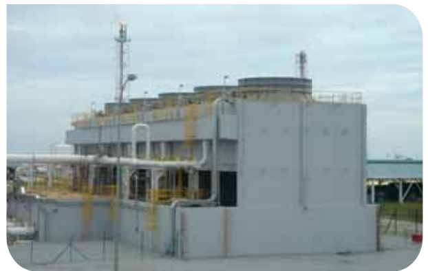
:: Malacca Cogen Power Plant, 12500 m 3 /hr (5 cells).
